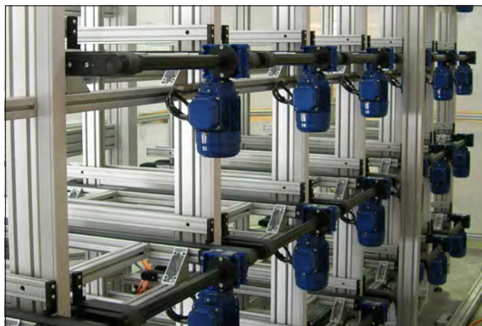
Double belt conveyor in a high complete automated storage
