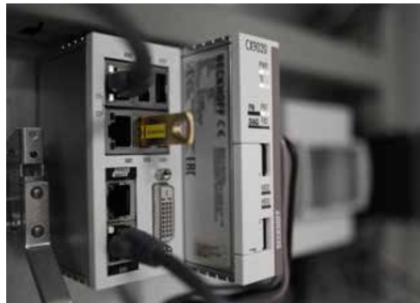
The Data Connection Extension Module of Hammer-IMS, a configured PLC system supporting Profinet, USB or OPC UA.
