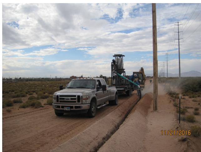
Figure 3. Production rates of 800 - 1000 ft/d were realised by the SAE automated delivery system.
