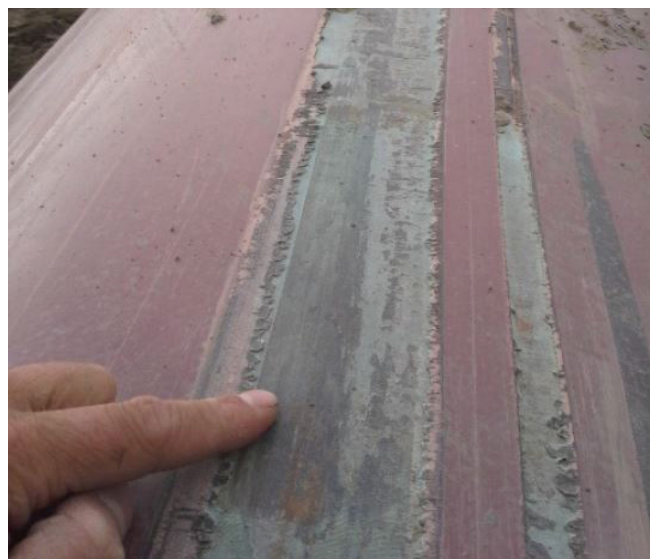
Figure 1. Scratch-like coating defects are likely to occur at HDDs.
