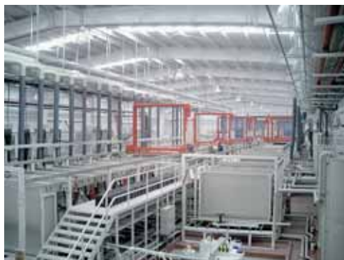
Abb. 1: Galvanisieranlage Figure 1: Plating plant
