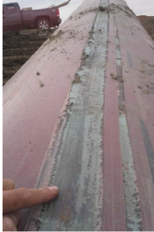
Figure 2 – scratch like coating damage observed during visual inspection
