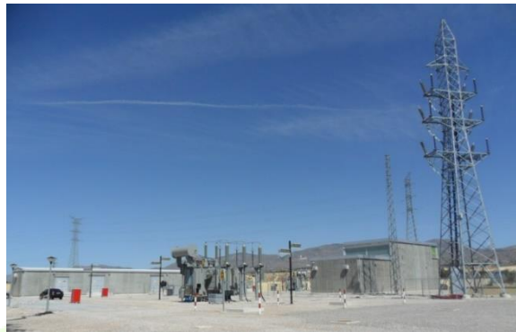
Figure 28 – Crevillent substation 132/20kV
