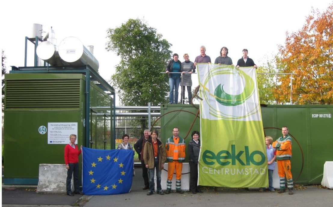
Figure 54 – Ecopower’s CHP on pure plant oil of Ecopower – Eeklo
