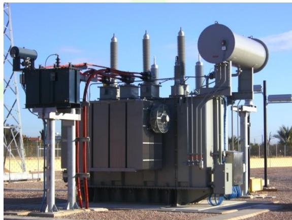
Figure 30 – 132kV/20kV 40MVA power transformer
