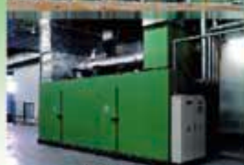
Combined Heat and Power
